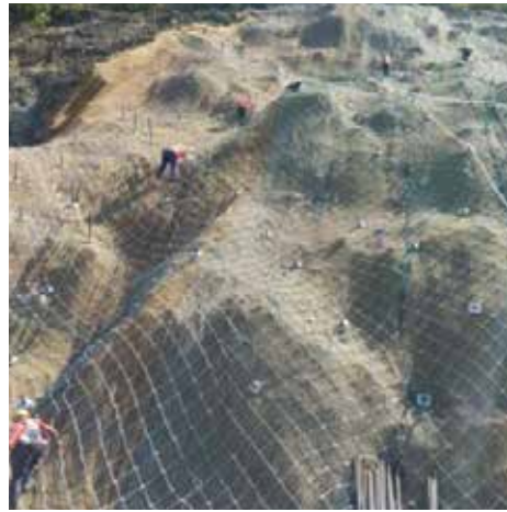
AFTER INSTALLATION OF HIGH STRENGTH WIRE MESH, COIR MAT, HYDROSEEDING & SOIL NAILING
